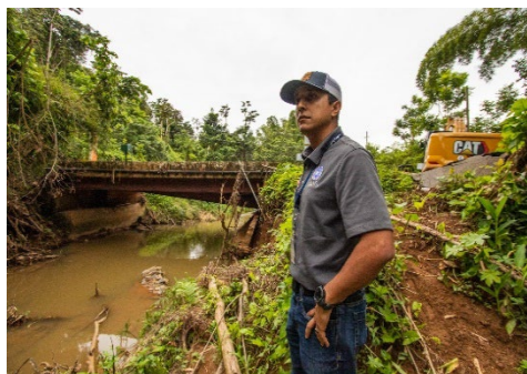
FEMA Operation Division Supervisor surveys a bridge that Hurricane Fiona severely damaged.
